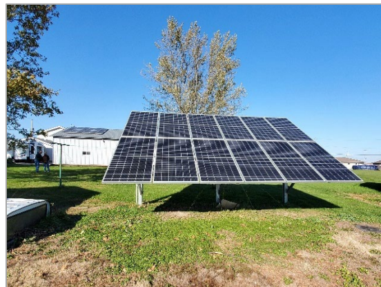
Residential Solar System in Springbrook Source: 2022 Jackson County Clean Energy Plan
